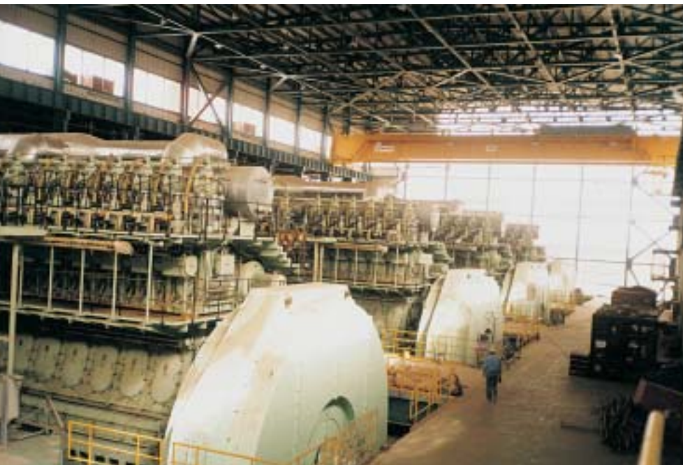
Severely damaged a short time before it could be commissioned, Hirgigo Thermal Power Plant was reconstructed with a supplementary loan.
